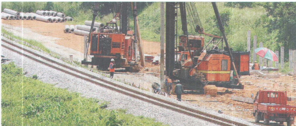
All systems go: Piling works being carried out for the electrified double-track rail project at Simpang Ampat in Nibong Tebal yesterday.
