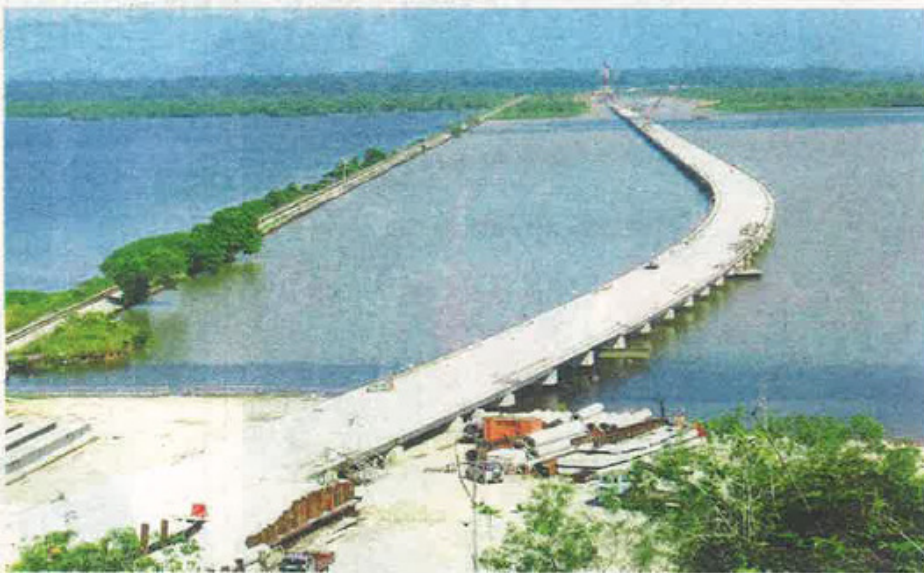
Work in progress: The 3.3km Bukit Merah Marine viaduct will replace the existing bund and allow free flow of water at the lake.
