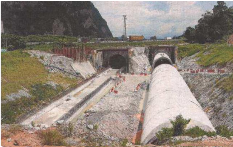
The construction of what is said to be the longest main line tunnel in Southeast Asia
