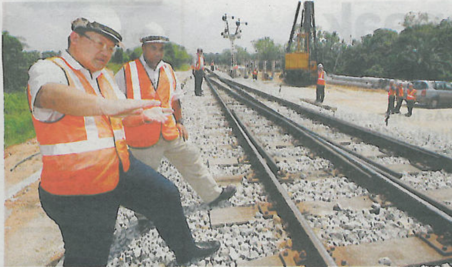
Site visit: MMC-Gamuda Joint Venture Project director (head of construction) Yeoh Hin Kok (left) and project manager Maslan Othman checking on the progress of the Ipoh-Padang Besar electrified double track project in Simpang Ampat, Nibong Tebal, yesterday.
